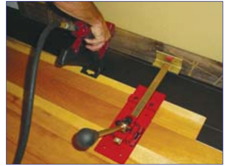
Using the PortaJack to tighten and lock a crooked board and hold it in place tightly, while fastening with the Portamatic 475.
